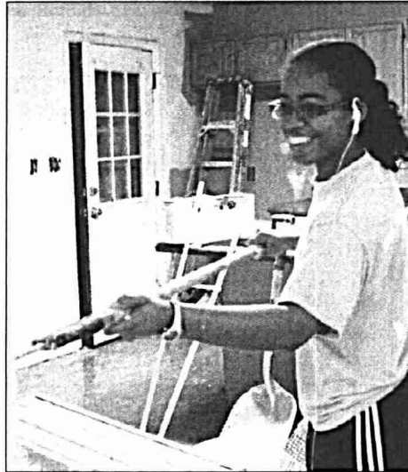
Mississippi College graduate student Otesa Wilson putting on a fresh coat of paint on a Habitat house on Glendale
